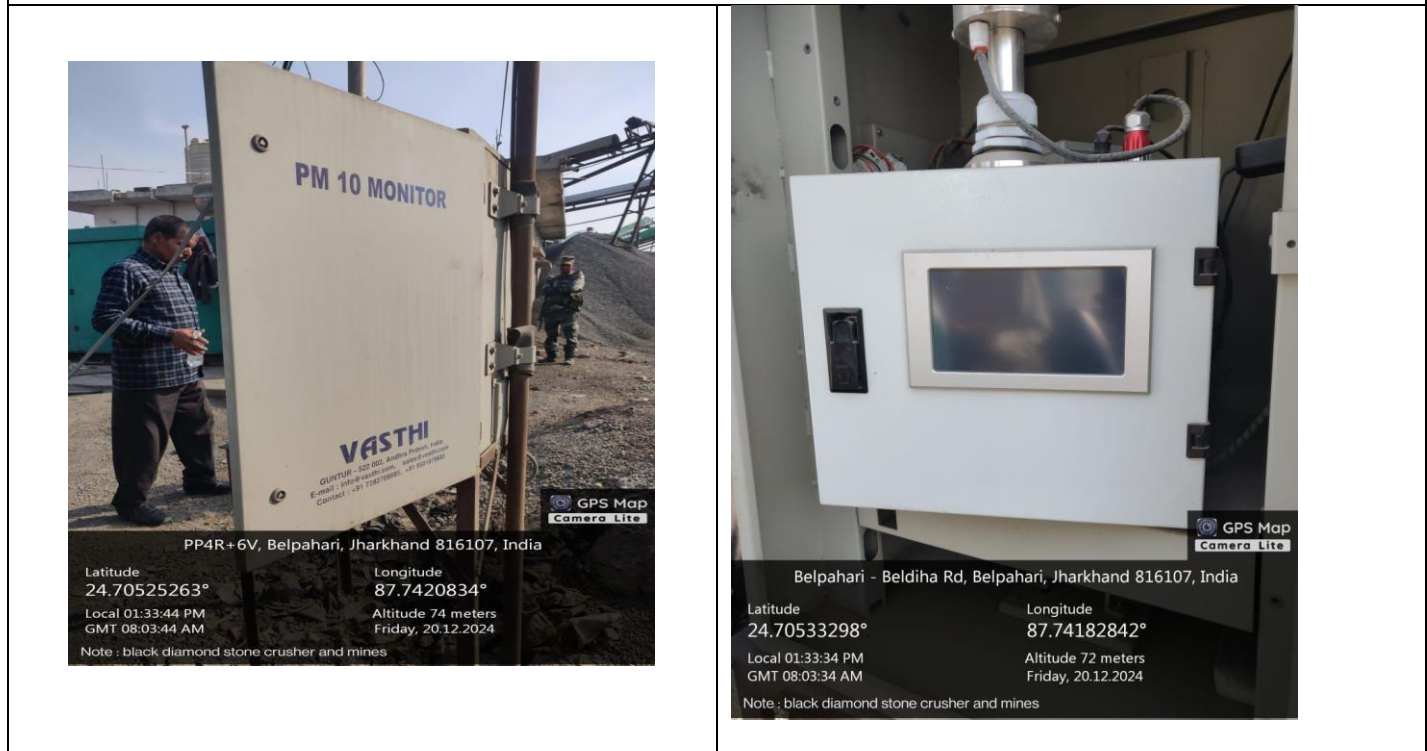
Figure 4: Photographs of the OCEMS device installed at M/s Black diamond which is offline and no data is getting transmitted to the JSPCB server
